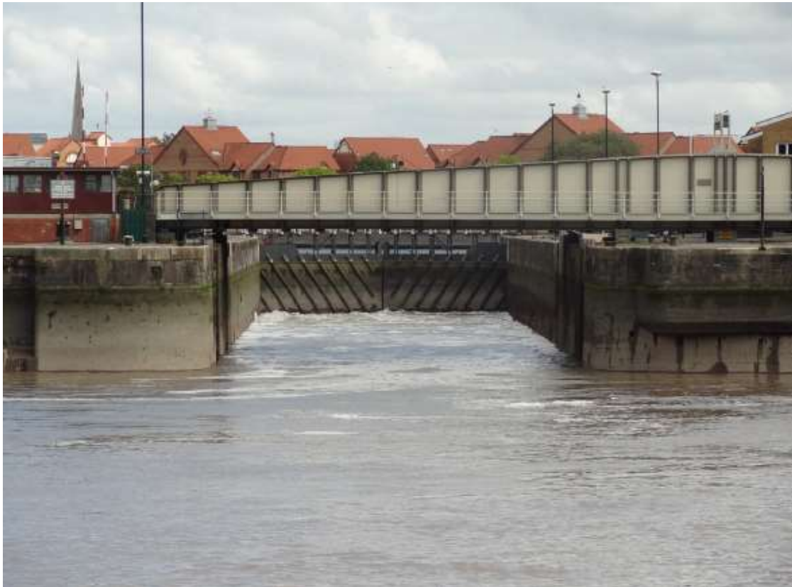
Plate 3 Junction Lock flood gates
